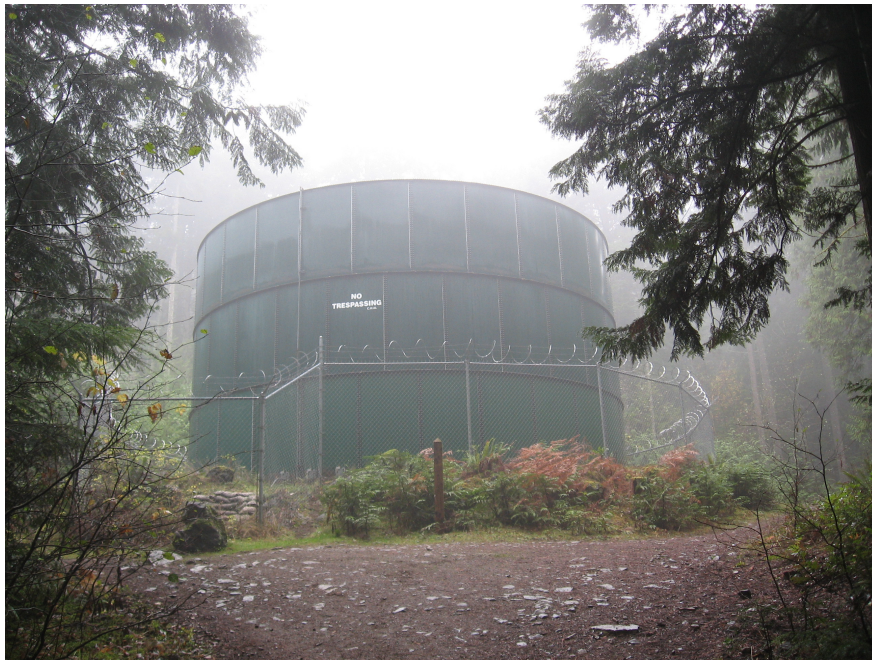
Cobble Hill Improvement District - 200,000 Gallon Reservoir
